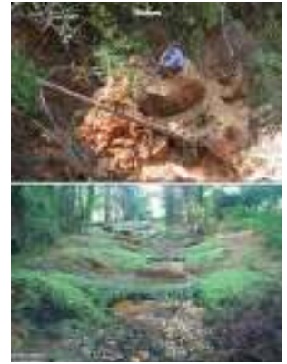
This before and after photo to the right shows the erosion on a tributary of Joe's Branch. Ashley Campbell with the City of Daphne sits on a boulder that fell off the wall of the stream after a storm last summer. The second photo shows a completed step pool conveyance in Anne Arundel County, MD. The restoration of the tributary of Joe's Branch will resemble the Maryland project.
